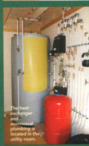
Radiators are connected at diagonal points - the most efficient way to connect a radiator. The thermostatically controlled valve is located in a convenient position for manual adjustment.
