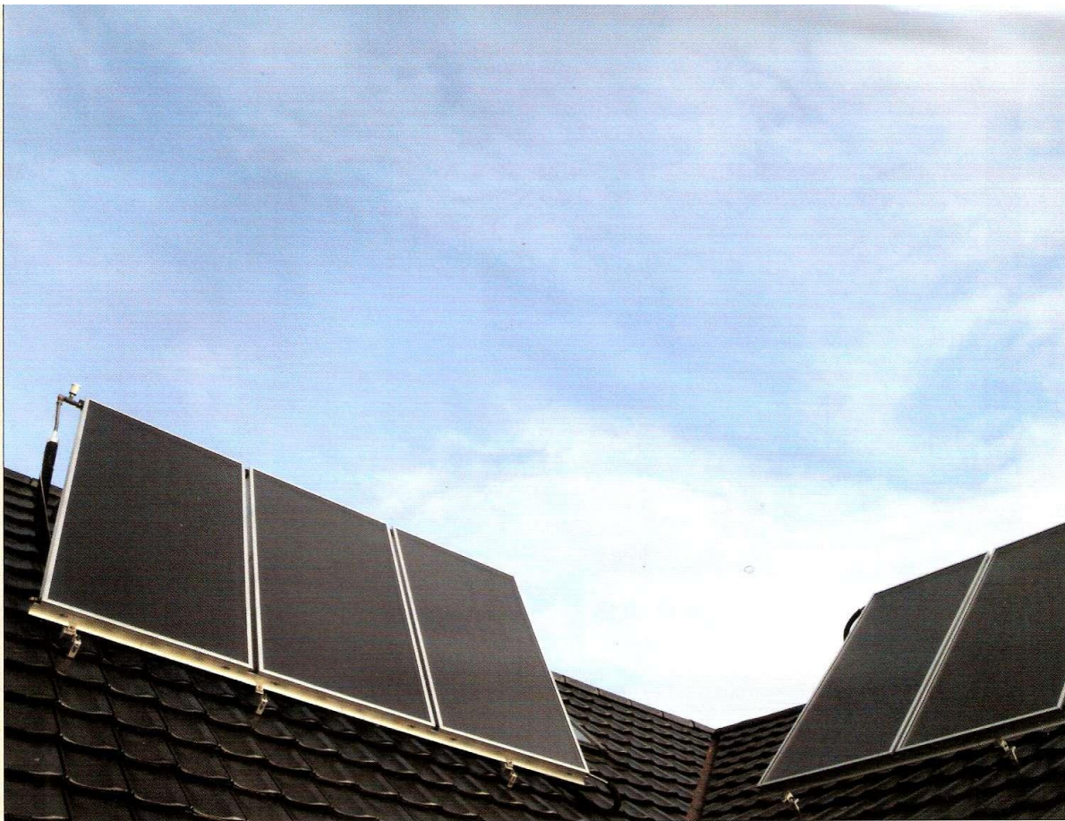
(above) There are a total of six solar panels on the roof and during the summer months the water temperature can reach 60 to 80 degrees by means of these panels alone; (next page) The Wamsler wood pellet stove, together with the solar, feeds a 1000 litre storage tank and a 140 litre expansion tank for water heating
