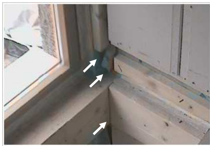
Figure 28 South West Corner Floor Level – Visible
